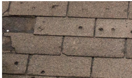
Large and fast-moving hail may compromise your roof structure's integrity.
