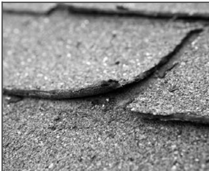
If shingles are missing, your roof is already close to failing.
