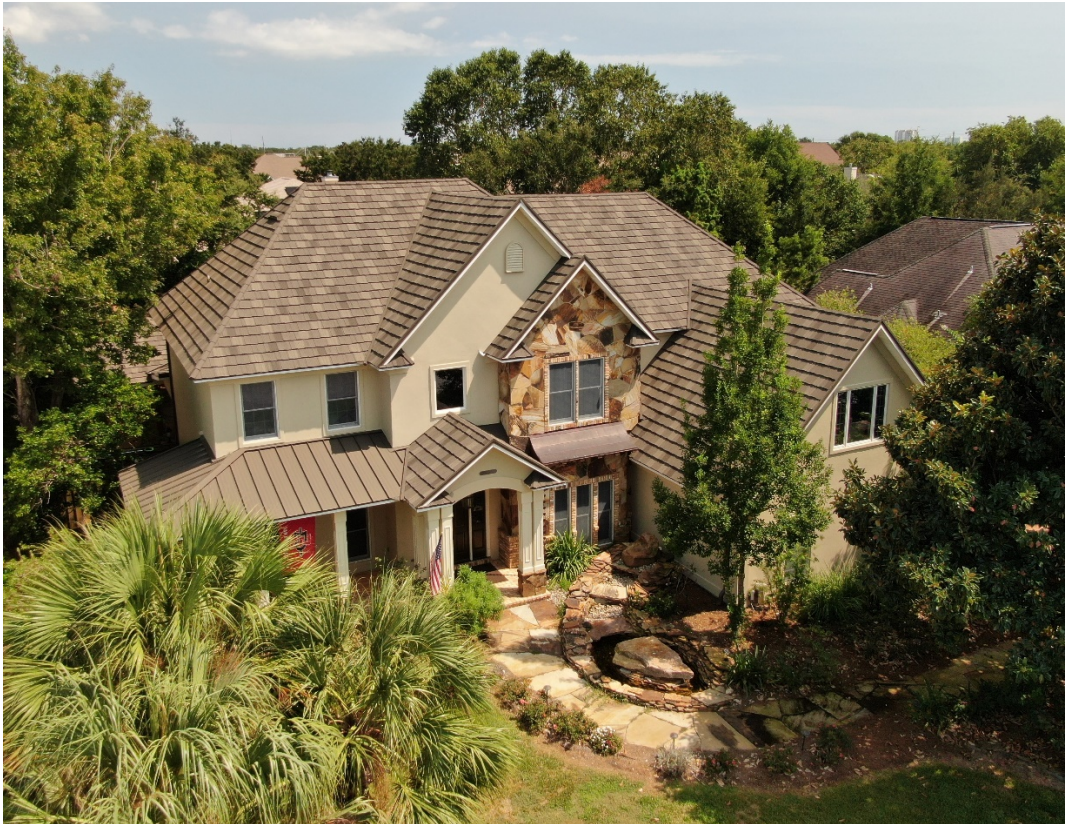
(Suggested image caption: A new DECRA metal roof installed by Weather Shield Metal Roofing in Gulf Breeze, Florida is the winner of MRA’s Best Residential Metal Roofing Project Competition for the first quarter of 2021)
